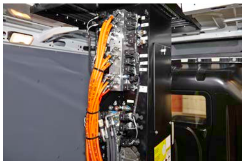
Ground level emergency lowering from the load area (pedestal mounted valve bank)
